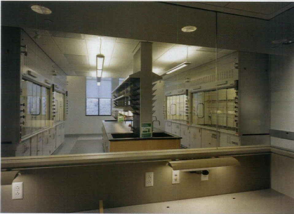
The north-facing laboratories have generous daylight supplemented by T5HO fluorescent pendants to meet Yale's requirement for an average of 75 footcandles on the lab benches (above).
