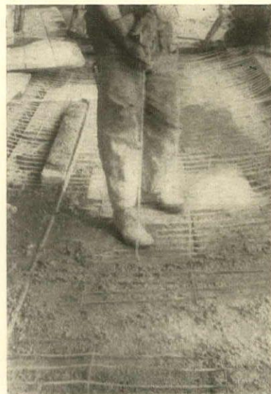
A lather pulls up the wire mesh so as to allow the concrete to cover its under side
