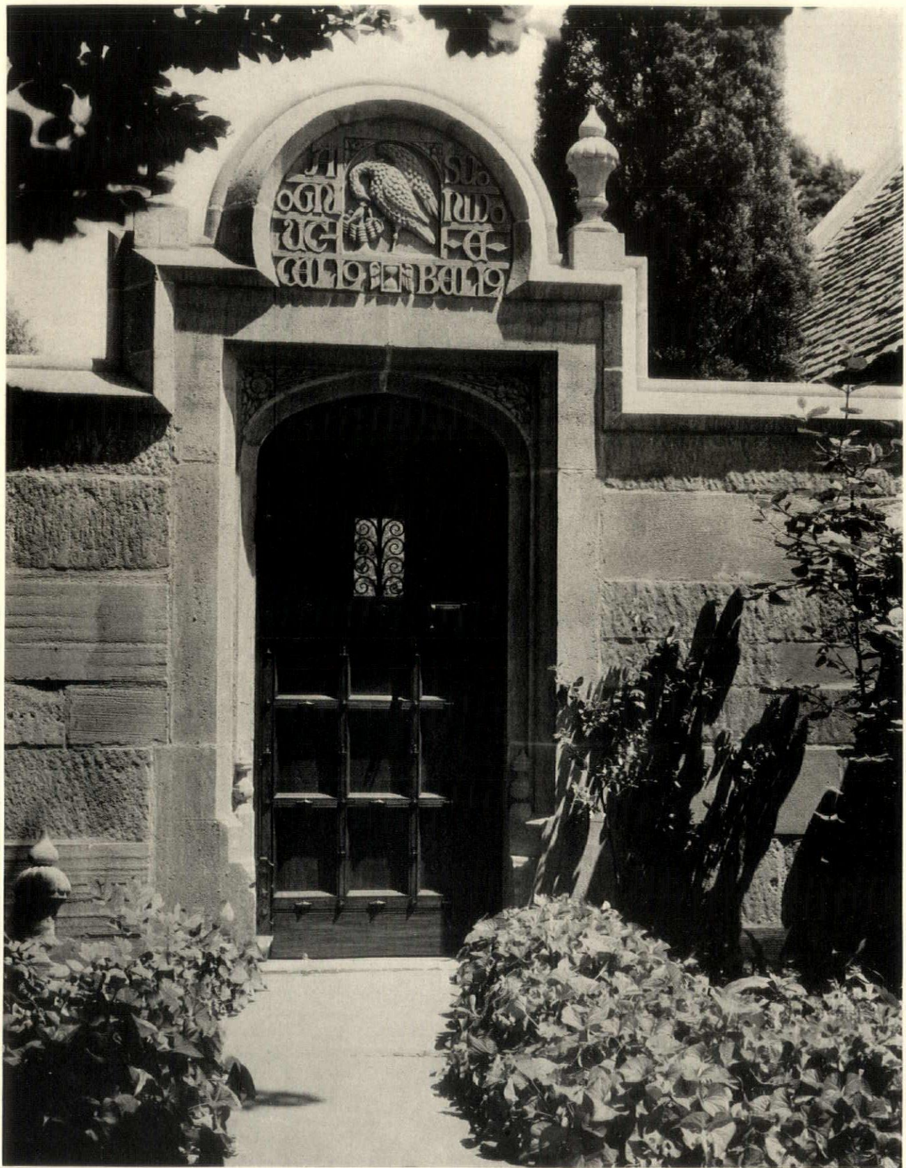
The garden gate in the east wall near the garage. A free translation of the inscription would be: "To every bird its own nest appears the most beautiful." This and the capping of the wall are of cast stone
