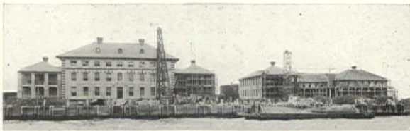
New Hospital Buildings at the U. S. Immigrant Station, Ellis Island, N. Y. All of these Buildings Rest on Raymond Concrete Piles.
