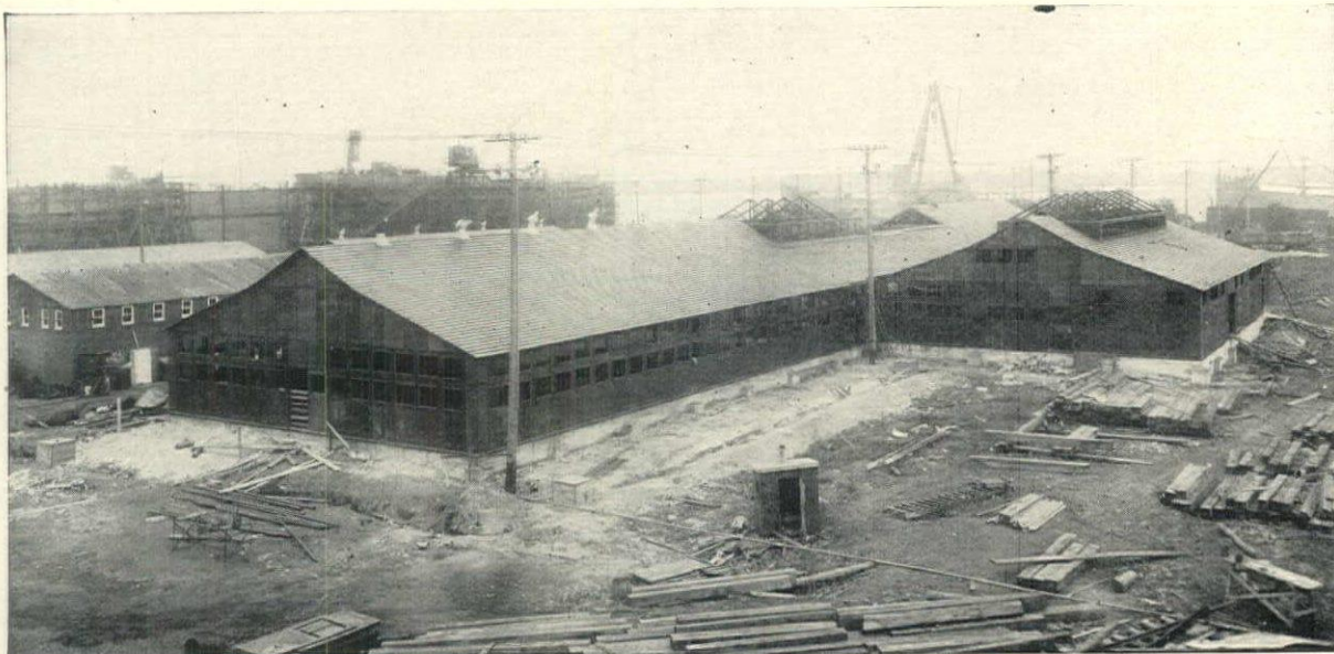
Construction of large dining hall and kitchen at Great Lakes Engineering Works, Ecorse, Mich. Smith, Hinchman & Grylls, Architects and Engineers, Detroit, had complete charge of the planning, details, construction and arrangement of these Truscon Steel Buildings.
