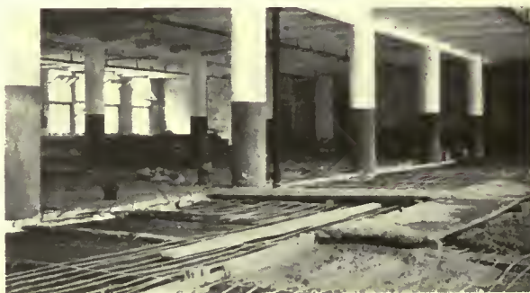
New slab being placed. Reinforcing rods showing are those taken out of demolished floor slab, straightened and re-used.
