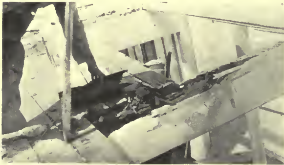
Fig. 9. Ends of roof planks rotted over the supporting beam. The rot has also extended three or four inches into the beam.
