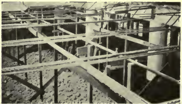
View looking down on first floor. False work for supporting forms already in place.
