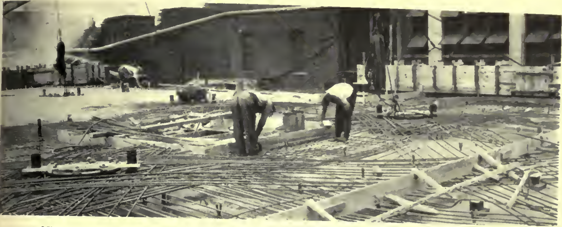
View of a partially poured concrete floor, showing the four-way reinforcing rods in place
