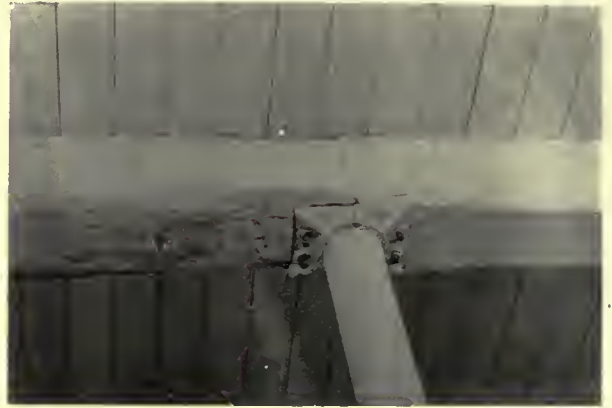
Fig. 18. Cast iron columns used as a drain pipe for rain water has precipitated water on and seriously rotted the beams which enclose it.
