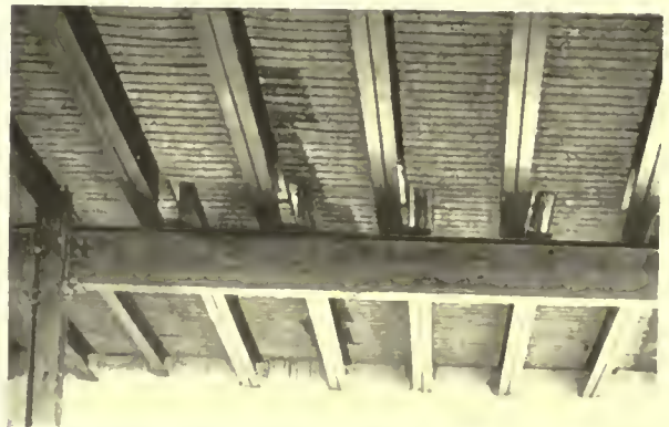
A floor with metal joists, structural steel girders and columns. Concrete floor slab in place. View from below.
