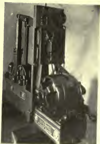
Motor driven pumping unit installed for Everett L. Brown
