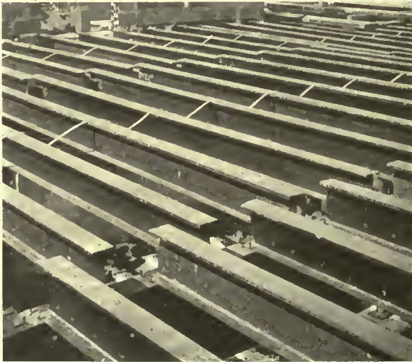
Floor construction in a large apartment house, metal joists supported on structural steel girders, galvanized iron bridging strips in place.
