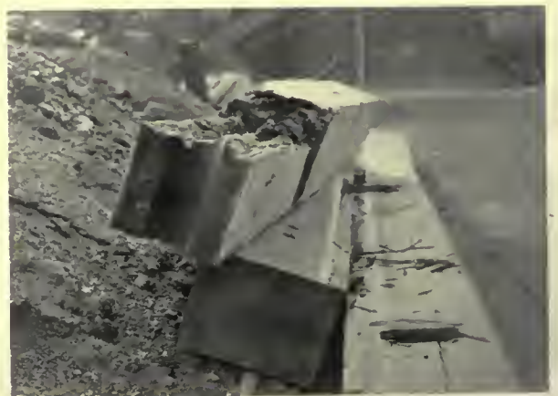
Fig. 19. Beam rotted for some distance from column, serving as rain water conductor, which it enclosed.
