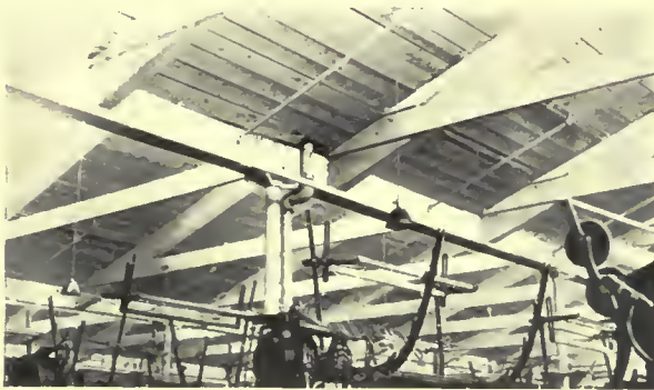
Fig. 17. This iron pipe, for carrying away rain water from the roof, has absorbed sufficient heat to precipitate water on the nearby roof, causing the roof to rot.
