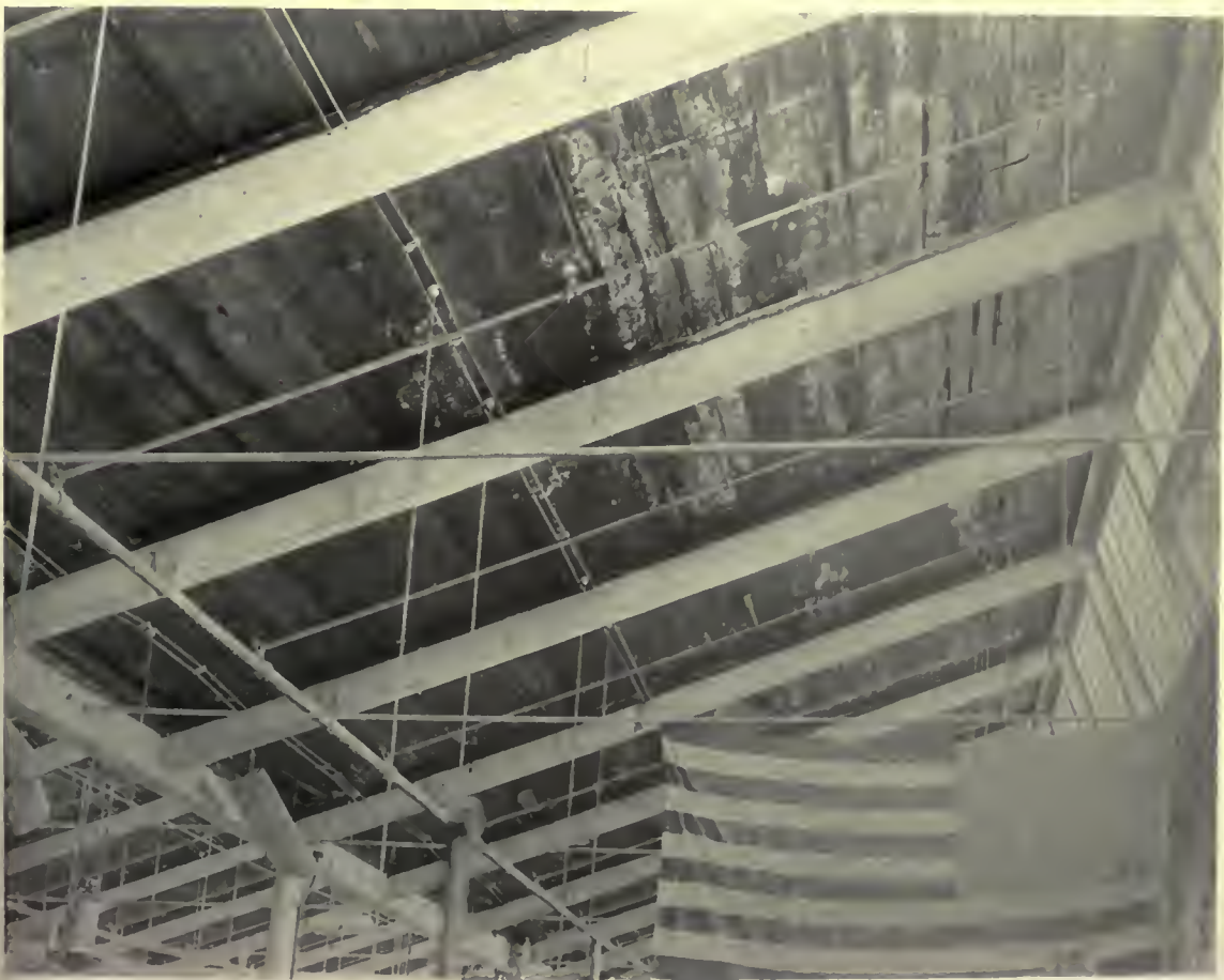
Fig. 15. Roof planks of a New Bedford weave-shed from which the sheathing has been removed. The planks were destroyed in nine years.
