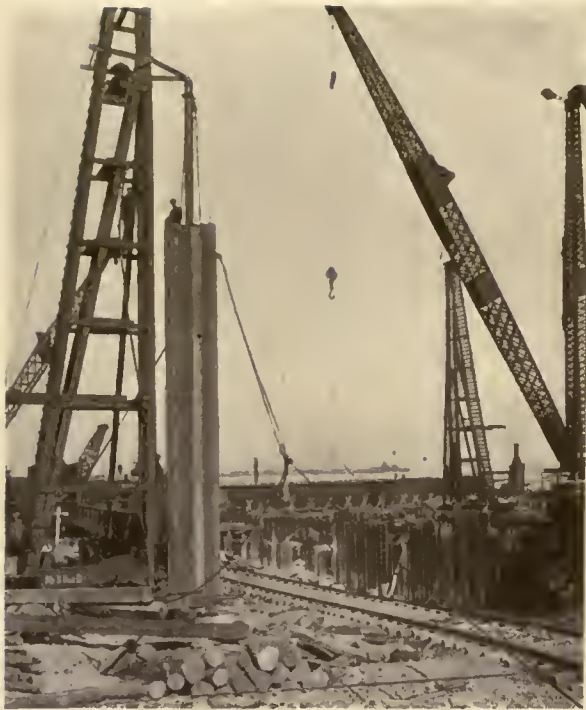
METHOD OF USING PILE DRIVER RIG Steel pipe holds cylinder of piling vertical for driving
