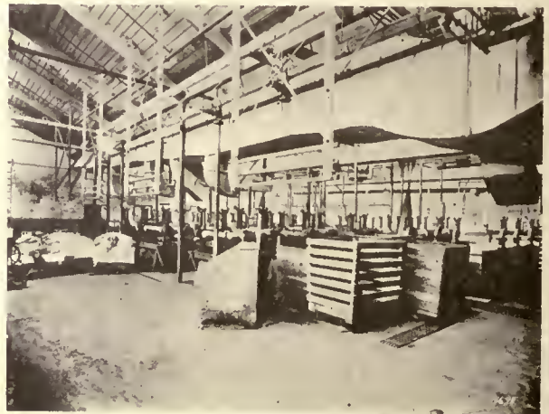
A DYE HOUSE INSTALLATION
