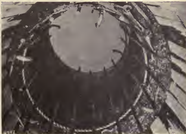
LOOKING DOWN INTO CYLINDER Rain water collects on top of concrete
