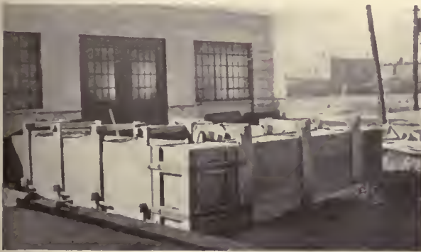
First Course—Shows form in place and filled with tamped earth EARTH HOUSE, ST. LOUIS, MO. THOMAS CRANE YOUNG, ARCHITECT
