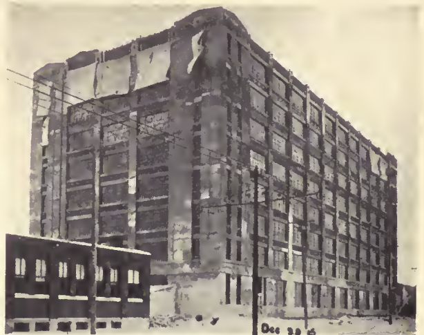
BUILDING FOR ROBERT SIMPSON CO., LTD., REGINA, SASKATCHEWAN. VIEW TAKEN DURING CONSTRUCTION
