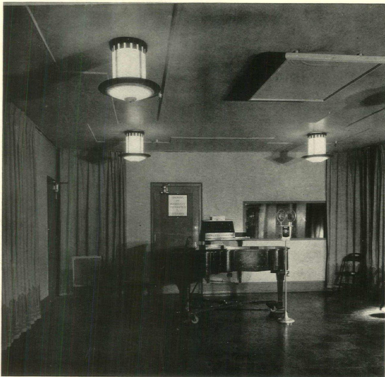
TYPICAL SMALL STUDIO SHOWING ANNOUNCER'S CONTROL BOX AT LEFT OF SOUNDPROOF WINDOW OF MONITOR'S BOOTH, VENTILATING EXHAUST, DUCT GRILLS, AIR DIFFUSER AT CEILING AND MOVABLE SOUND ABSORBING CURTAINS ON TRACK
