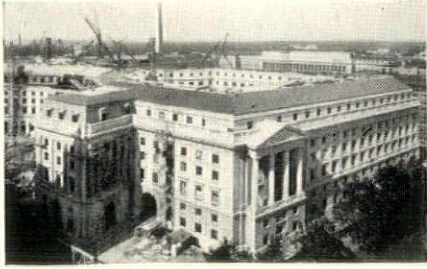
POST OFFICE BUILDING. Contractor, Mehring and Hansen. "Freon" air-conditioning equipment by York.
