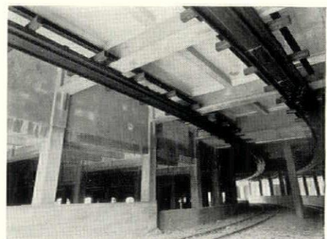
Subway under new Rundel Memorial Library. Entire lower slab, beams, and suspended pipe spaces, as well as all radiator recesses in building, were corkboard insulated by Hunkin-Conkey Construction Company.
