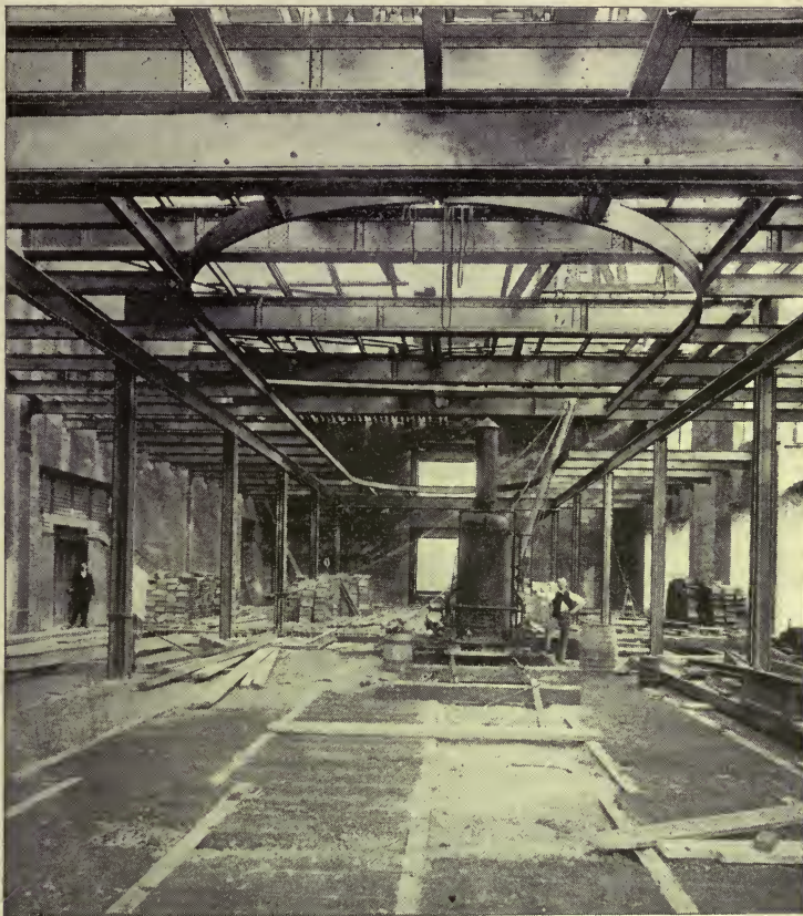
Riveted girder and hoisting engine, new wing, American Museum of Natural History.
