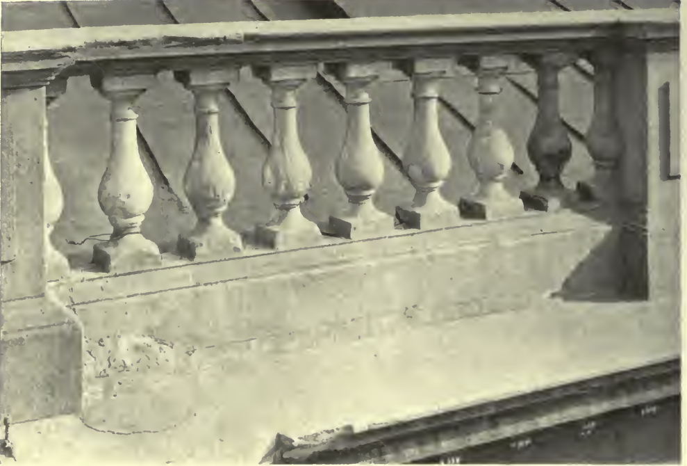
DETAIL OF BALUSTRADE ABOVE ROOF, SHOWING PREVAILING CONDITION OF MARBLE—NEW YORK CITY HALL.
