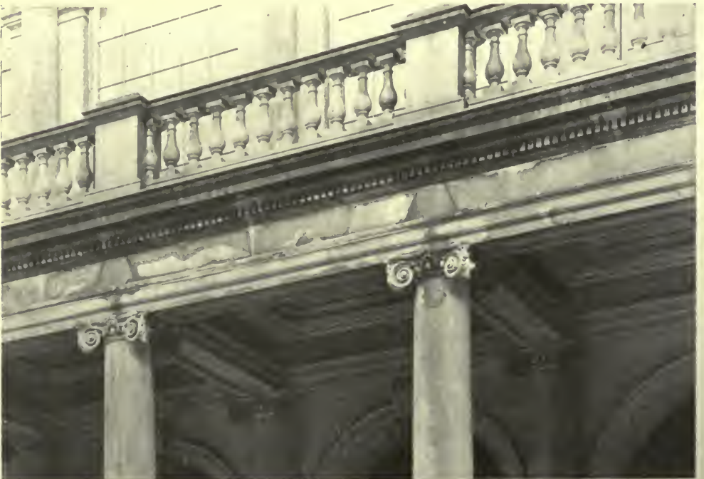
DETAIL AT PORTICO—NEW YORK CITY HALL. COMPARE THE DETAILS OF THE OUTER COLUMN CAPITALS WITH THOSE THAT HAVE BEEN PROTECTED BY THE ROOF.
