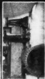
These 10-inch Jenkins Standard Fire Line Valves, Range, with rising spindle installed in kitchen line.
