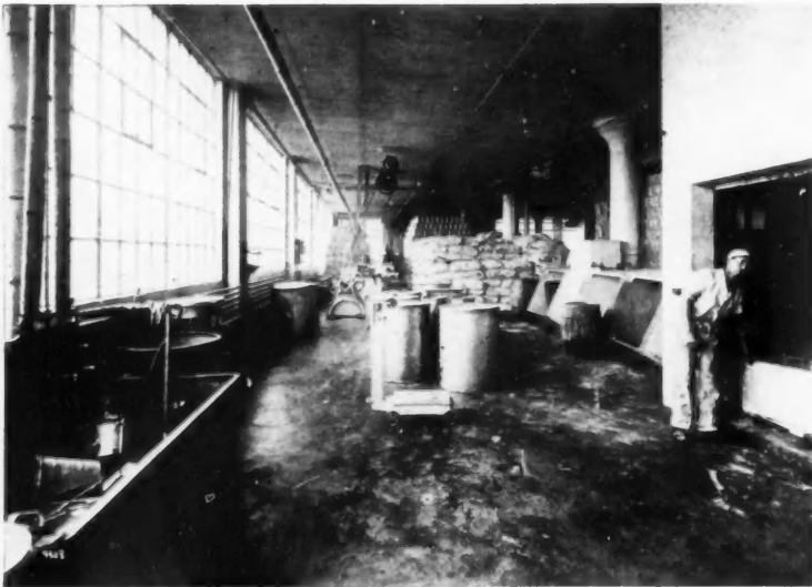
The floors in many plants and warehouses are continually covered with substances that cause and accelerate disintegration of the concrete. The condition pictured here is commonly observed.
