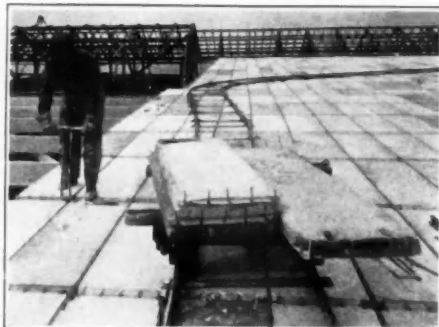
Method of tying Gypsteel Roof Slabs to give roof definite, computable, structural strength
