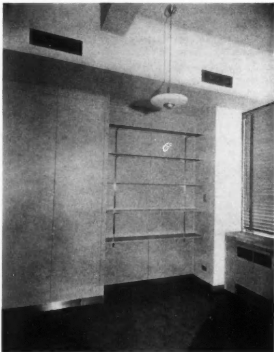
Air conditioning grilles for office space in the new Philadelphia Savings Fund Society Building (Howe and Lescaze, architects). Each floor of this bank and office building is controlled separately for the conditioning of air.
