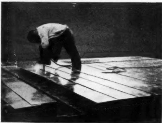
A LIGHTWEIGHT STEEL FLOOR with strength attained by shape and welding of units.
