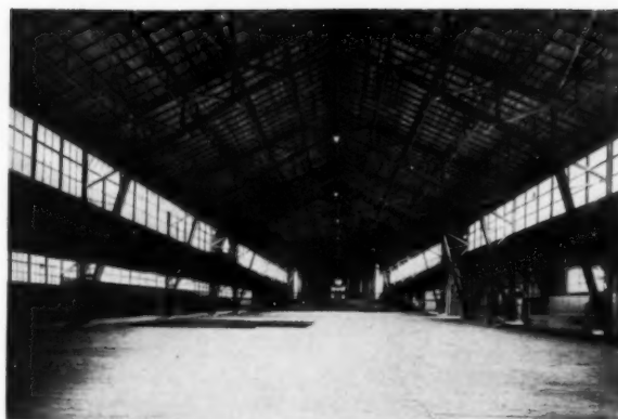
Exhibition hall at Ludwigshafen, Germany. Modern connectors used for all joints of three-hinged 100-foot wood trussed arches spaced 41 feet apart.
