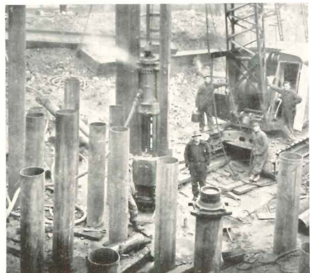
Even before being filled, this piling tested as high as 92 tons per pile.
