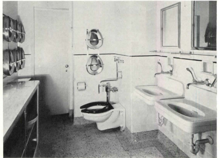
Service room for two four-bed wards, Chicago Lying In Hospital.
