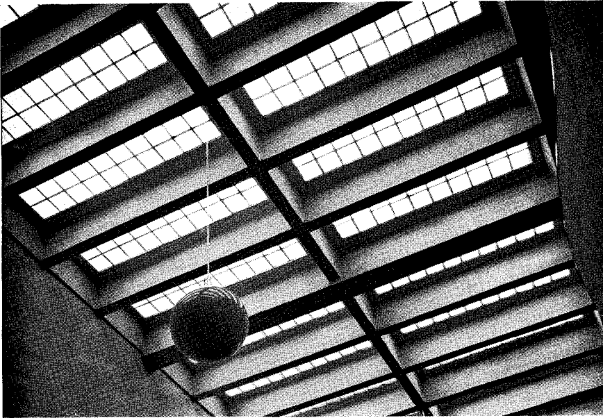
Detail of ceiling skylight. The reinforced members were poured in place. Sash are steel; glass is opaque for diffused light.
