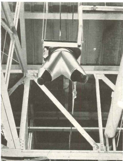
SPLITTER DUCT on heater outlet
