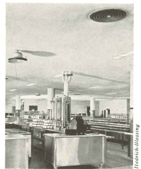
CEILING OUTLETS, factory cafeteria
