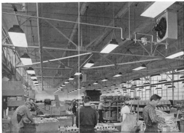
While many modern installations use fluorescent lamps in continuous rows, with this type of lamp it is possible to achieve good even lighting with fewer fixtures placed at fairly low height
