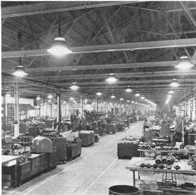
Combination mercury installation. Each unit uses one 250-watt high-intensity mercury lamp and three 100-watt incandescent lamps. It provides 20 foot-candles upon working surfaces
