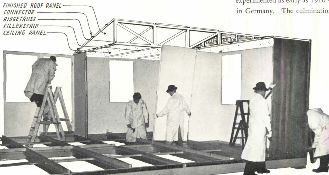
Assembly of small house, fitting exterior wall-panels in place at corner; also interior partitions, before finished floor panels are installed
