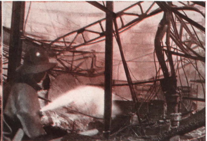
Aircraft parts were made in this "fireproof" building - until fire struck leaving it a mass of twisted metal.
