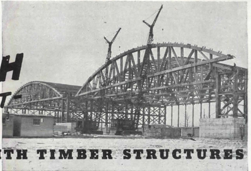
CLEVELAND. 200' laminated trusses were designed, prefabricated and erected by Timber Structures, Inc. for 200'x440' assembly plant, for The U.S. Engineers. Front trusses, (supporting doors and roof), were built to carry 450,000 lbs. Intermediate trusses built to carry 310,000 lbs.
