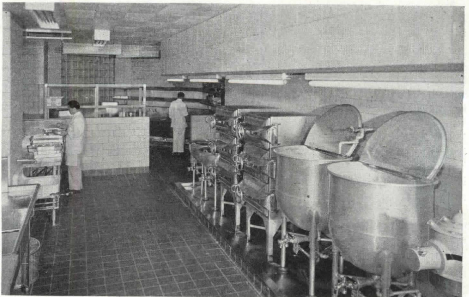
Vegetable section of main kitchen (second floor) has metal-faced acoustic tile ceiling, glazed brick walls, tile floor
