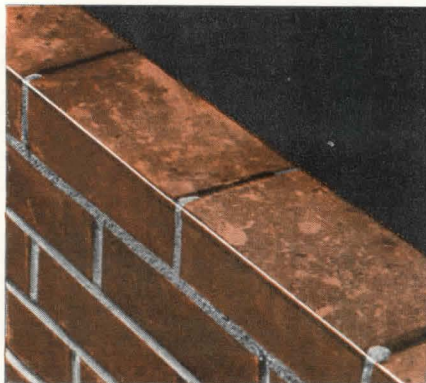
the mortar does not fill the head joint.
