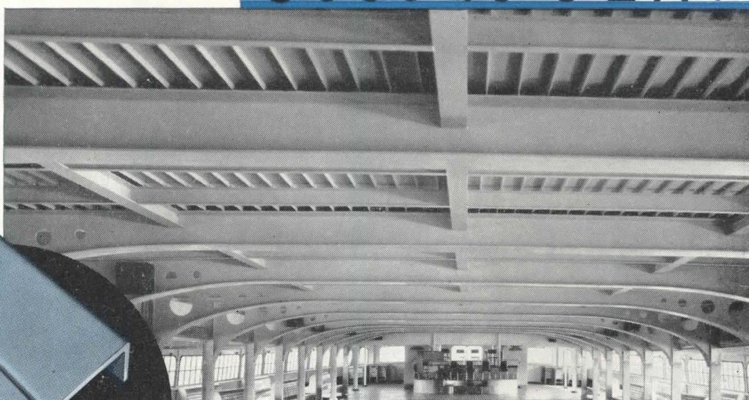
The Decks of the "Delaware Belle", new Wilson Line Excursion Boat, are of Mahon Steel Deck rolled from Yoloy.
