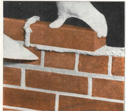
So that the mortar oozes out at the top of the head joint.
