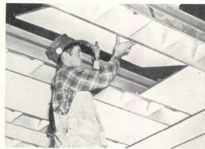
Panels of acoustical Fiberglas fit between light troffers to form a suspended ceiling
