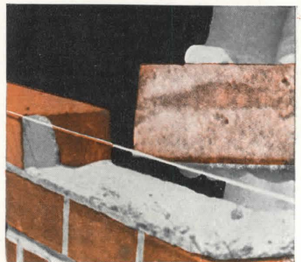
Only part of the head joint is filled with mortar.
