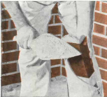
Plenty of mortar should be thrown on the end of the brick to be placed.
