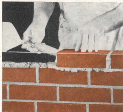
So the mortar dried out too much before the next course of brick was placed on top of it.
