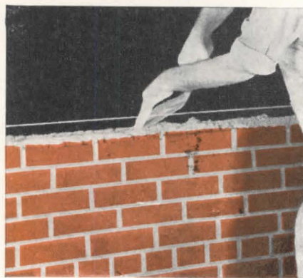
Mortar for this bed joint was spread out on the wall too far.
