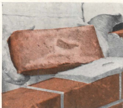
Therefore the mortar did not stick to the top brick. A good bond was not secured.
