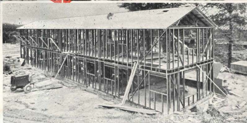
Construction view of Stran-Steel framework for first unit, Kent Village Apartments. Roberts Construction Corporation, owner and contractor; Berla and Abel, architects.
