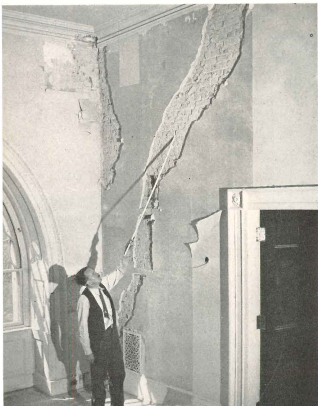
Plaster has been removed from one of the brick partitions to show settling cracks; these walls have no footings, were never intended to bear present loads
