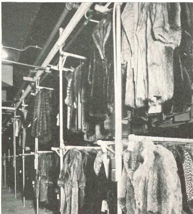
Proper spacing of furs in the vault is essential for good ventilation. (Photo courtesy Abbott, Merkt & Co., Engineers)
