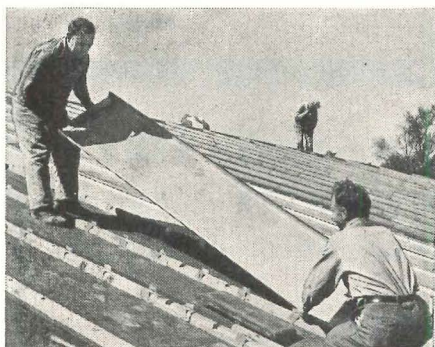
INSTALLING MONEL BATTEN PANS over wooden batten bars. The pans have pre-formed ends that provide watertight joints without solder. Monel nails and cleats are used to lock the pans and the Monel batten caps together.
