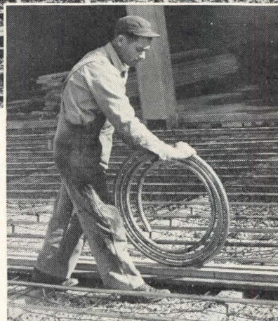
GUIDE PLANK is used by workman to facilitate installation of 1" Type K soft temper Revere Copper Water Tube. Revere Tube also comes in hard and soft tempers in straight lengths of 20 ft.
