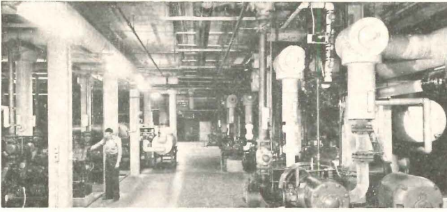
Machine room in Merchant's Terminal warehouse. Refrigeration equipment of York manufacture totals 245 tons capacity and uses "Freon-12" refrigerant.
