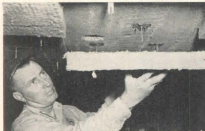
Insulating Walls and Ceiling by Miracle Surface Anchor Method. Fibreglas insulation, Type PF-613, 2" thick — bonded to concrete ceiling using Miracle Pronged Anchors. (Illustration: Radio City Studio 3B, New York, N. Y. Contractor, William J. Scully, Inc., New York, N. Y.)
