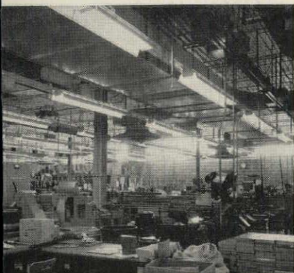
"NECK LINE" High efficiency, all-purpose fixtures with upward component of light to give severe brightness contrast. Ideal for Machine Shop and Factories .
