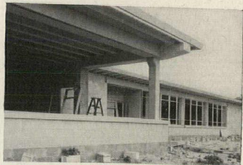
Rear view of classroom building shows variety of units used—concrete block, precast columns, cantilevered beams, window beams, lintels and cantilevered roof channels.
