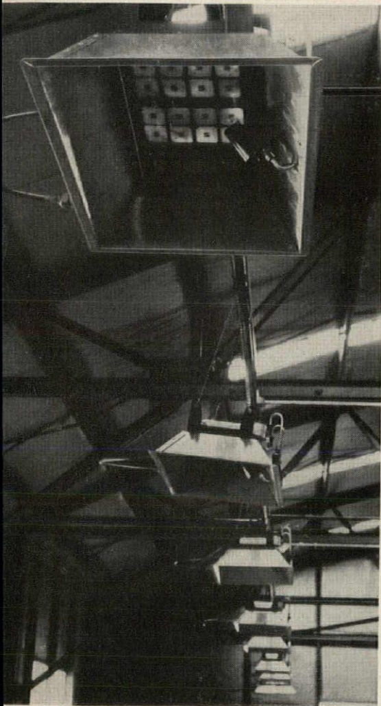
Closeup shows typical generator, with ignition, gas supply and control relay
