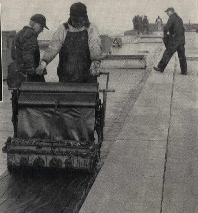
Three Jobs in One Pass. This Lexsuko applicator applies non-flammable Lexsuko Adhesive R907T to the underside of Koroseal Vapor Barrier, lays and secures the Koroseal, and places ribbons of adhesive on top of the Koroseal for securing insulation—all in one easy operation.
