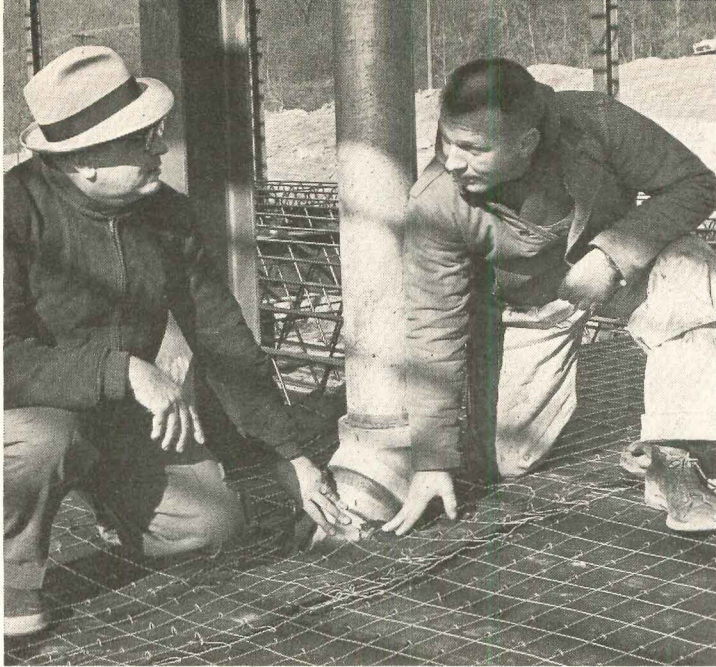
Snug fit of Steeltex around drain pipe at Canevin High School is shown by Joseph V. Cutuly, job superintendent (l.), and Foreman Dean Regan. Mr. Cutuly says, "Steeltex takes more punishment during installation than a sheet material, goes down faster and is much easier to handle."
