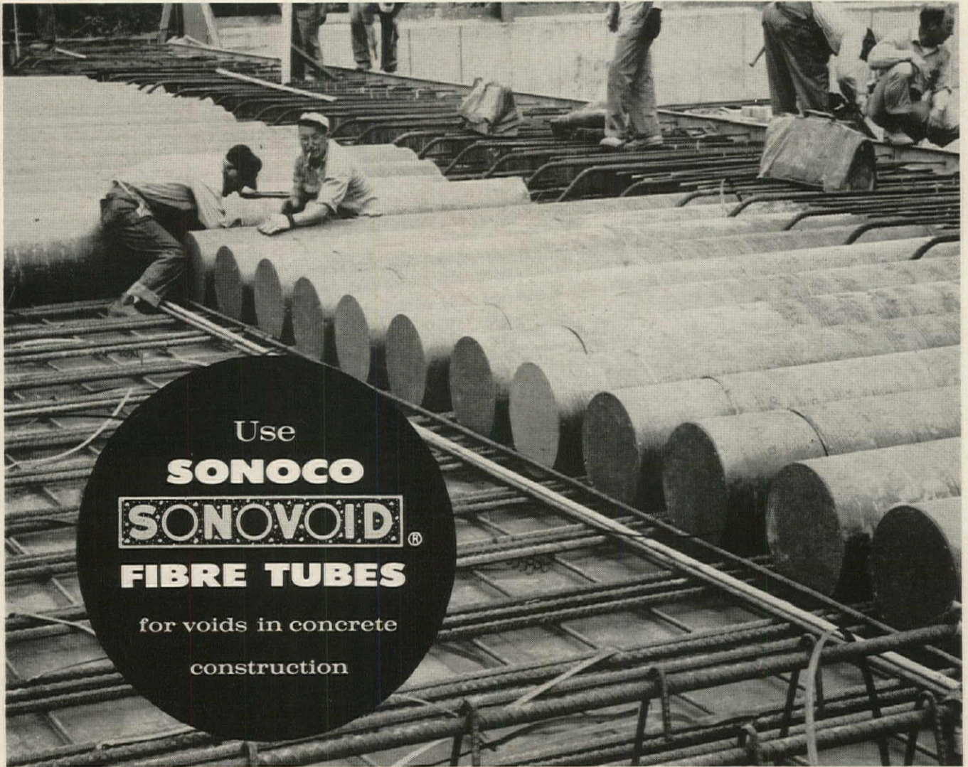
Homewood Flossmoor Community High School, Flossmoor, Illinois Contractor: Edward Gray Corp. Architect: Perkins & Will
