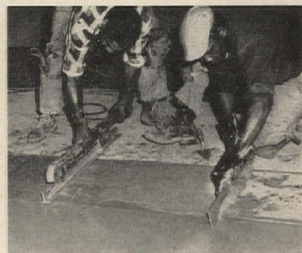
A "hot straight edge" is used to finish epoxy floor. Heat draws epoxy to surface giving finished floor high luster
