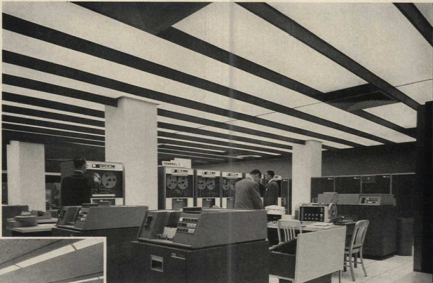
IBM DATACENTER — CHICAGO, ILLINOIS
