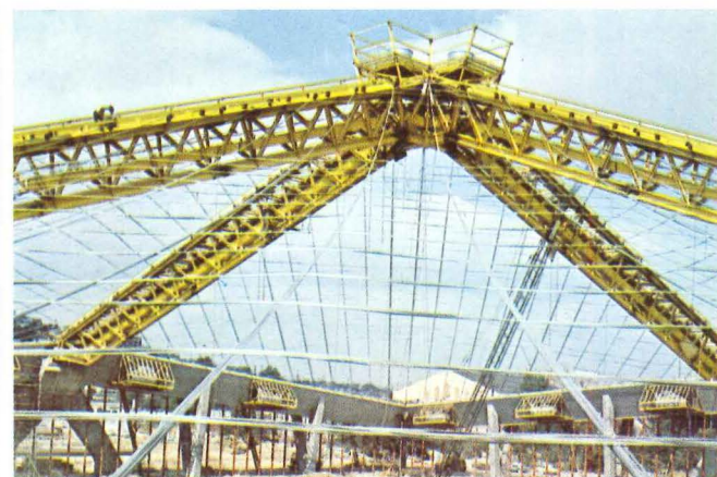
Unusual Coliseum building will enclose three acres of unobstructed space, rises 110 feet at the center. Four concrete tripods act as abutments for steel compression trusses between which are laced steel cables to form hyperbolic paraboloid roof. Cables will support the roof panels. Architect: Paul Thiry, F.A.I.A.; Structural Engineer: Peter Hostmark; General Contractor: Howard S. Wright Construction Company; Fabrication and Erection: Isaacson Iron Works. All of Seattle, Washington.
