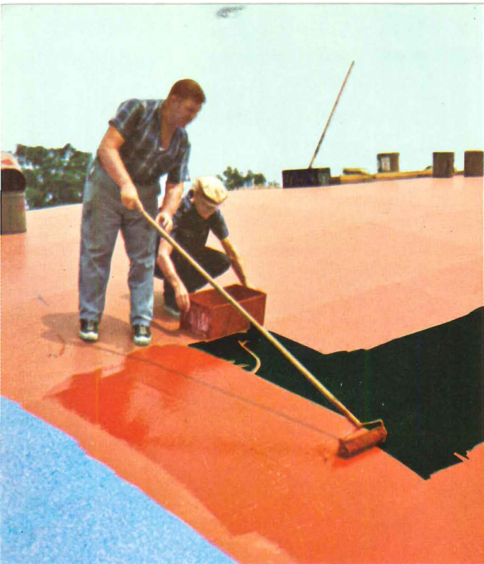
Application of F/A Roofing involves five basic steps. Mechanics here use the roller method as they apply the second coat of F/A 400.
