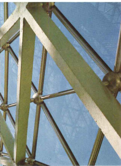
Glass, metal and concrete unite in a geometric masterpiece of skylight construction. Again glass demonstrates its ability to contribute dramatic impact while achieving functionality.
