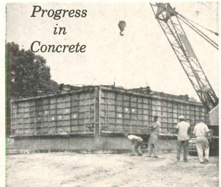
Progress in Concrete A complete form for concrete house being lifted by crane. The unit, of Symons Forms, has 5,000 square feet of surface.
