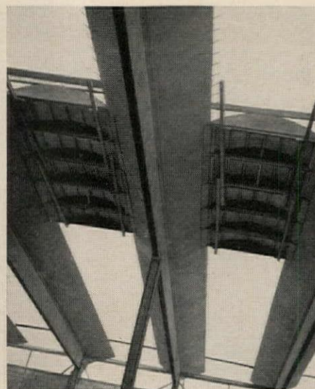
To complete the interesting form of the roof, 8' wide parabolic arches are poured-in-place between the beams.
