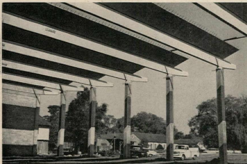
Eight prestressed Y beams are set in place on 16' centers as the first step in roof construction. Each beam measures 105' long and 8' wide.
