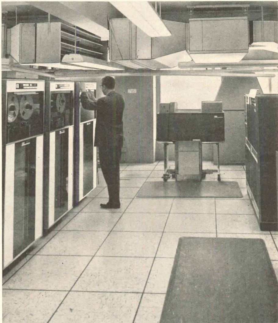
MELVILLE SHOE CORP., New York, N.Y. The computer room in this shoe company headquarters is air conditioned by a York "packaged" unit that maintains the temperature and humidity levels required for efficient computer operation. Contractor, Penguin Air Conditioning Corp., Brooklyn, N.Y.
