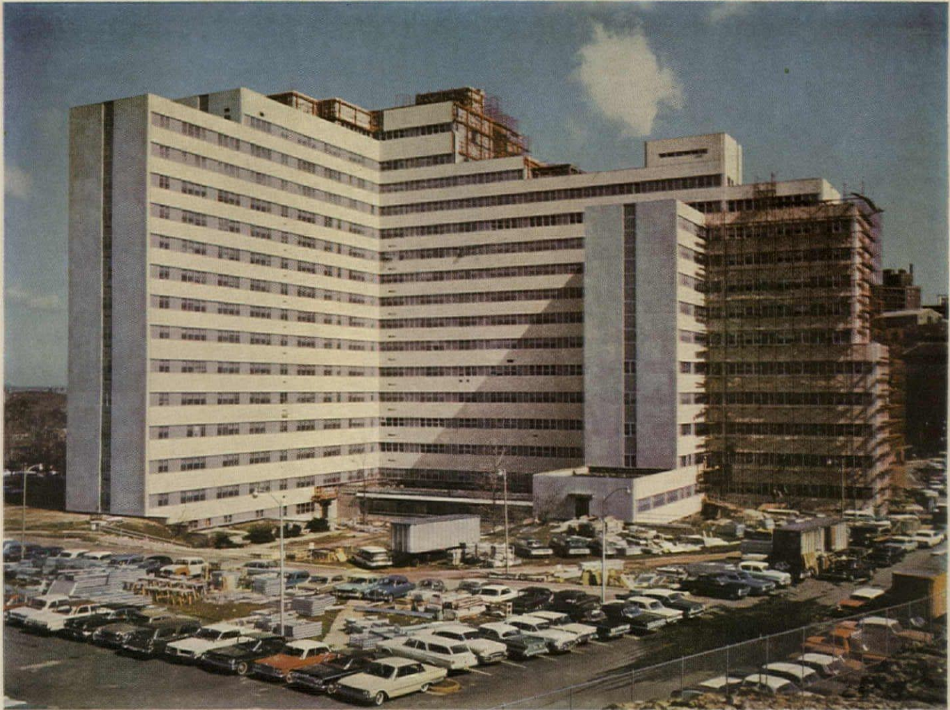
Over one million bricks were replaced by Plasteel aluminum panels while the hospital continued its day-to-day operation.
