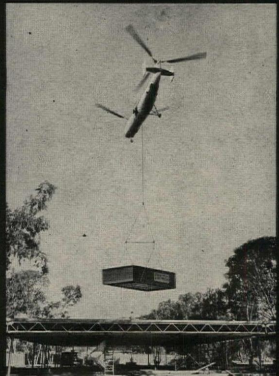
First of 400 Lennox 16-ton DMS cooling units being installed on prototype building of Ford Foundation SCSD project in California.
