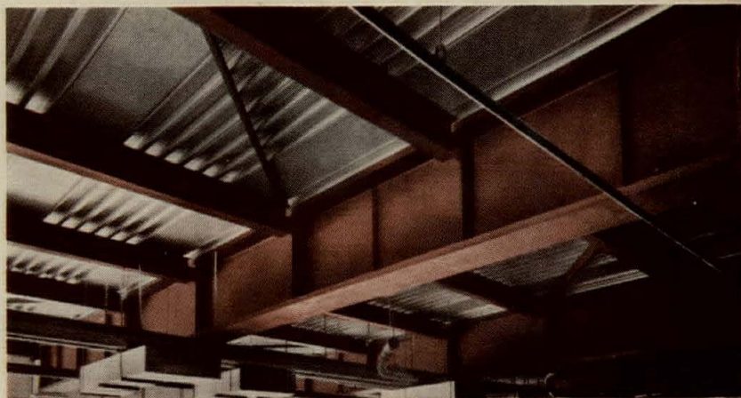
Two 36-in. deep girders of USS "T-1" Steel, 19 feet apart, saved two feet of headroom making 49-foot clear span possible.
