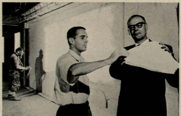
M. Tulou, who supervised installation, and owner B. Gordon examine cured urethane foam section from wall surface.
