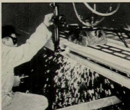
Primed steel can be cut without adversely affecting corrosion resistance when zinc-rich primers based on EPON or EPONOL resins are used. The zinc fuses around the cutting area as in hot-dip galvanizing.
