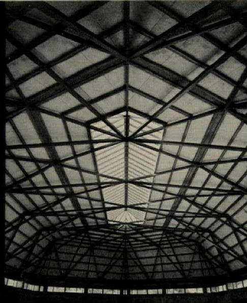
At the springing directly above the window strip, the space-frame roof creates an eave, then proceeds in a series of planes to the central skylight.
