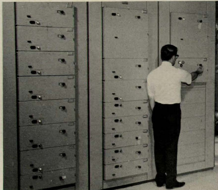
Main distribution panel, with pull-out type switches serving various sections of the 246-unit apartment project at Kenilworth.
