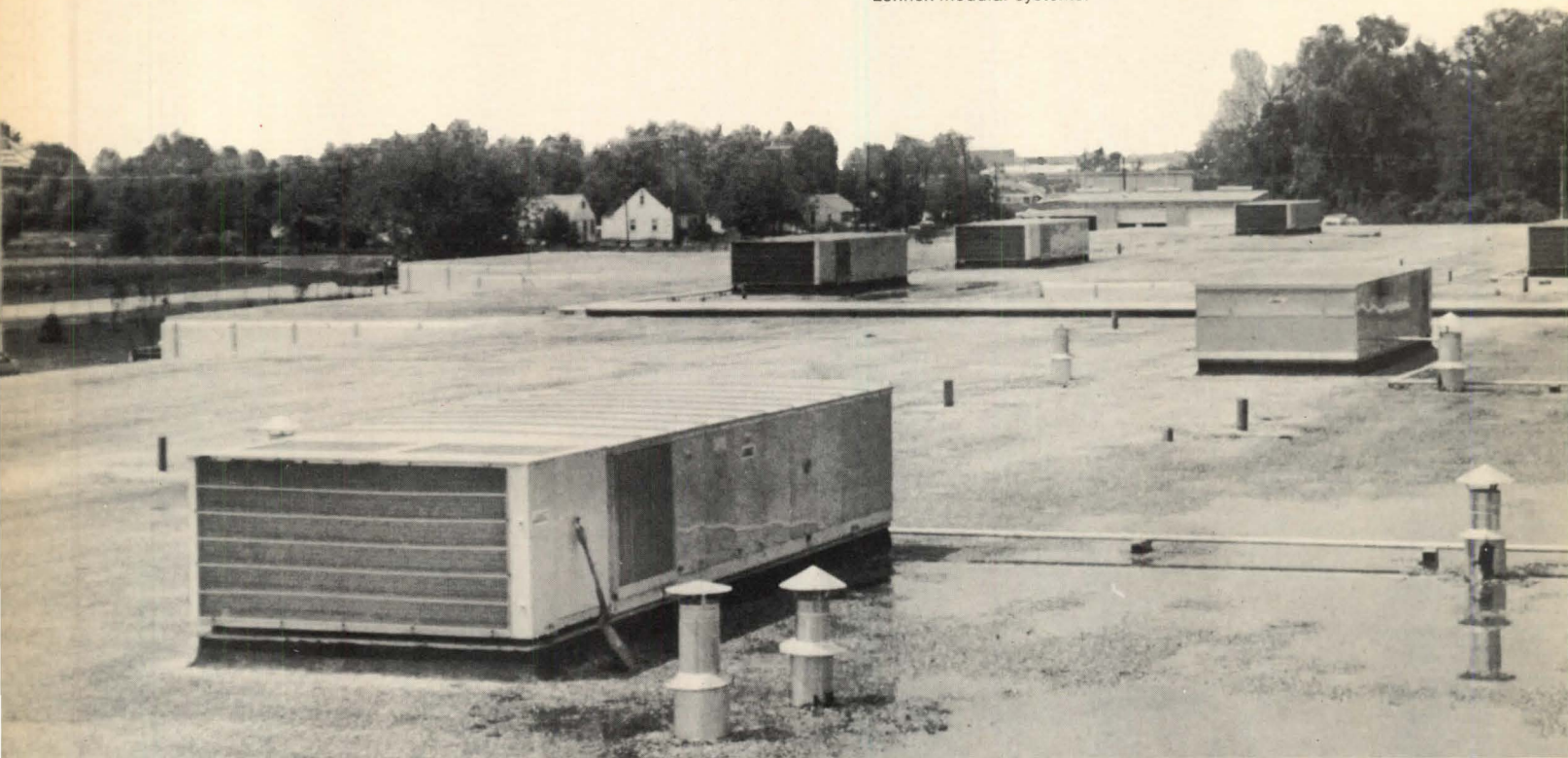
Kerr employee comfort and laboratory-accurate temperature control are both provided by Lennox rooftop DMS units. Eleven such units have a total output of 192 tons of cooling and 5,350,000 Btuh heating. Twenty-three other Lennox modular units supply supplementary heating and make-up air. POWER SAVER™ equipment on DMS units provides free cooling when outdoor temperatures fall below 57°F.
