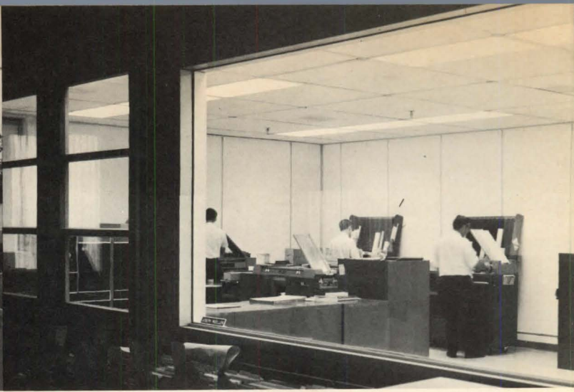
Careful planning is shown by Kerr's data processing room, with underfloor cable space for future equipment. Such rooms are isolated—but with broad expanses of glass for a "wide open" feel. The necessary "micro-climates" are provided by DMS and other Lennox modular systems.
