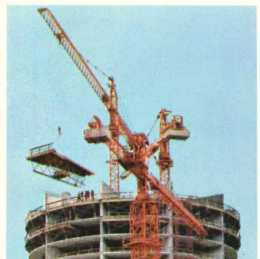
Peachtree Center Plaza, Atlanta, GA A Western International Hotel Developer: Portman Properties Architect: John Portman & Associates General Contractor: J. A. Jones Construction Company
