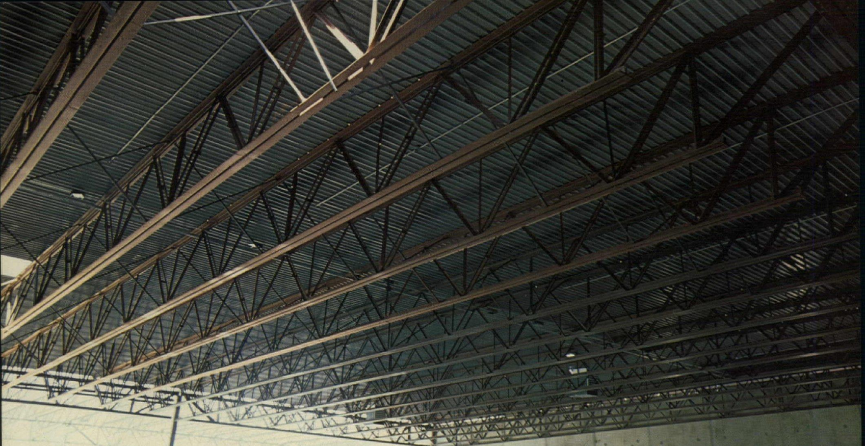
Long-span joists of 106' length provided large clear span bays needed for this building.
