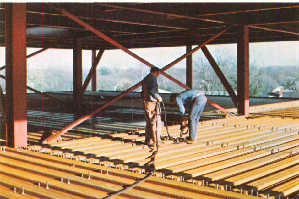
The floor system consists of a 3/4-in. lightweight composite concrete topping over 2-in. non-cellular composite steel deck. Floor-to-floor height is 12 ft. Bethlehem furnished all of the structural steel requirements for the building.
