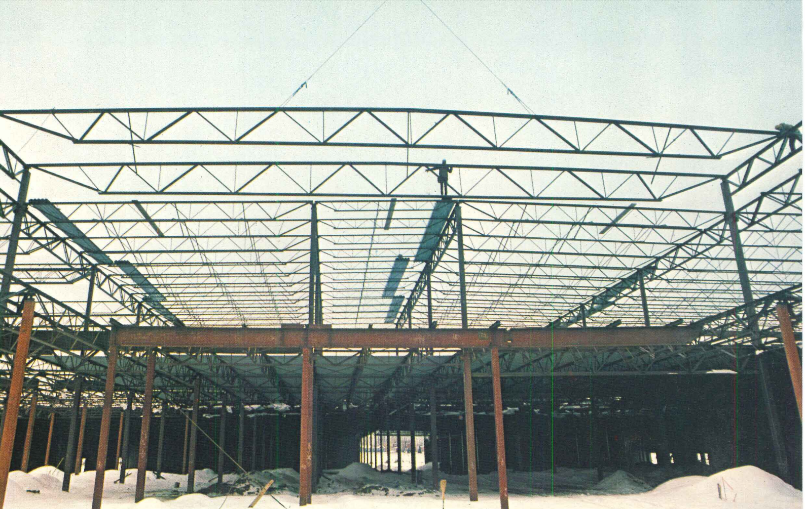
Use of 100' long span joists and 30' joist girders created a large clear span area in the center section of this enclosed shopping mall.
