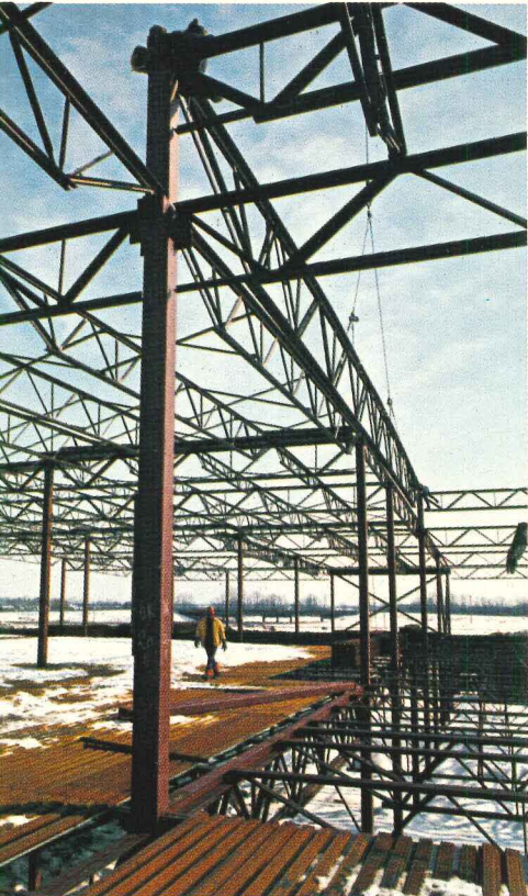
Wide spacing of deep steel joists (8" in floors and 7'6" in roofs) resulted in stiffer floor system and saving in the cost of joists.
