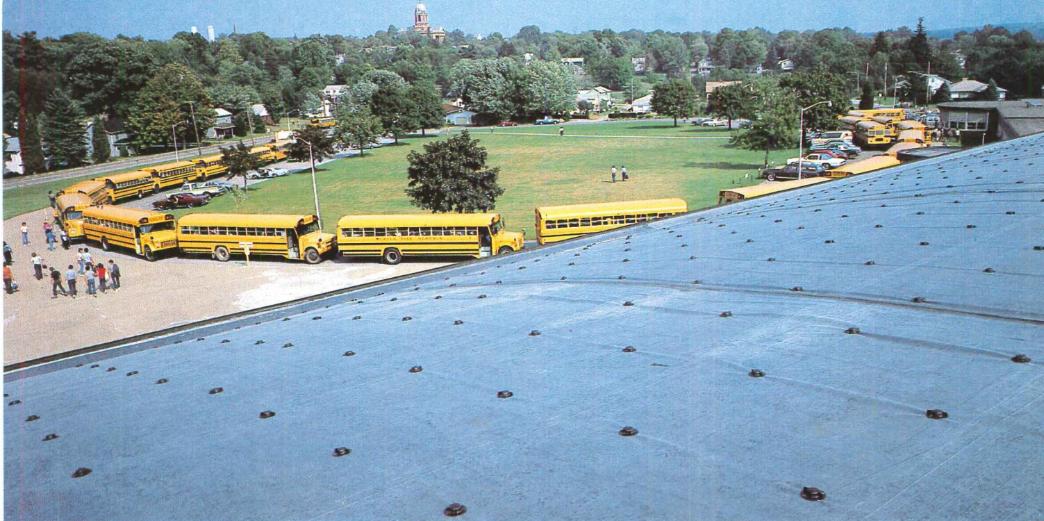
The Mercer Area High School, Mercer, PA Roofing Contractor: J.A. Burns & Sons, Mercer, PA
