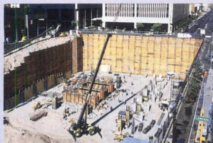
Two Renaissance Square, Phoenix, AZ — 483,000 Square Feet Above Grade—453,000 Square Feet Below; including a portion of the structure constructed under an existing street. Owner: Trammel Crow Company Architect: Pierce Goodwin & Alexander General Contractor: McCarthy Western
