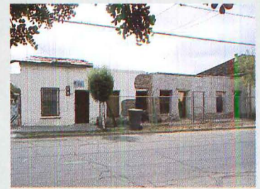
An old adobe wall (above) was restored as a freestanding entry (top) using traditional lime plaster. Existing openings were used for a new door, gate, and windows.
